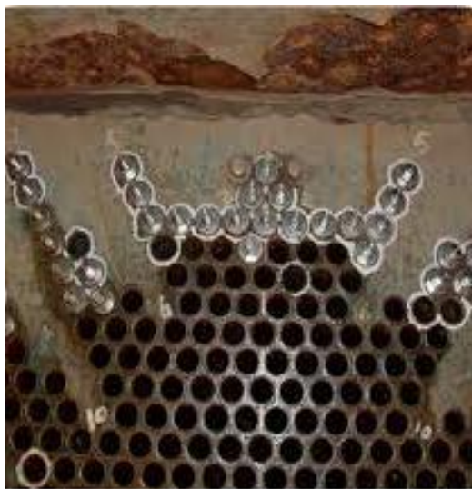
Figure 3 - Leaking tubes are identified and plugged
