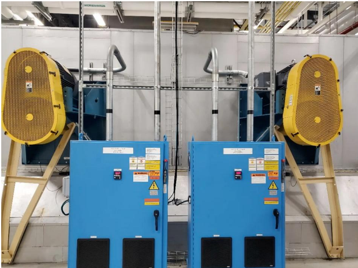
Figure 1 – Supply Fans being monitored by the LUBExpert ON-GUARD
