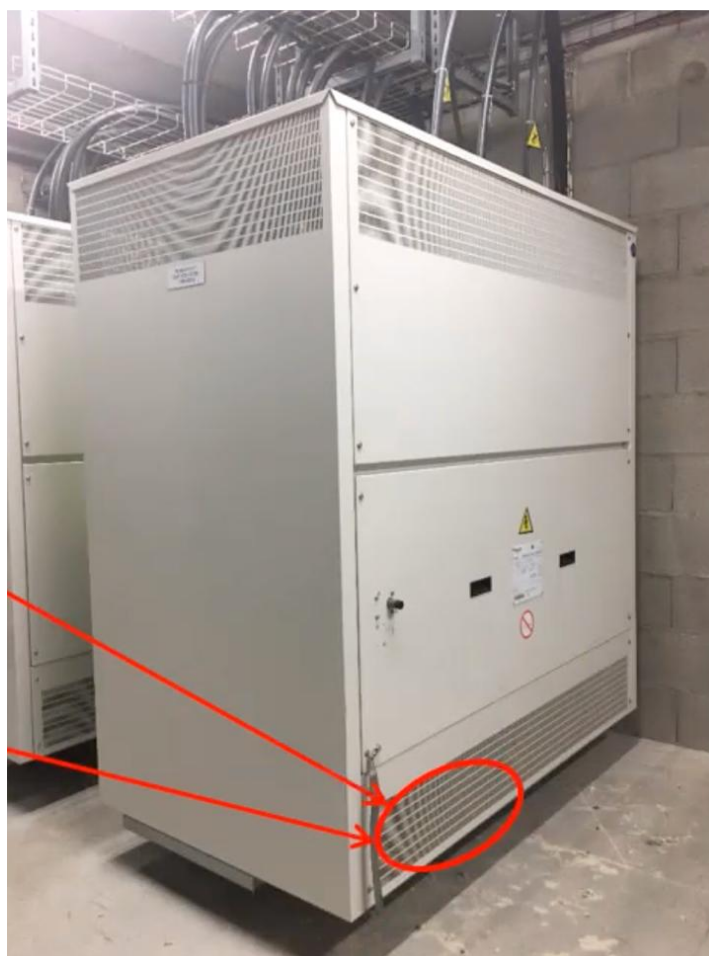
Figure 1 – Transformer in Question, highlighted is the area where the technician found the fault.
