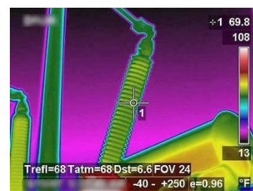
The thermogram showed no hot spot.
