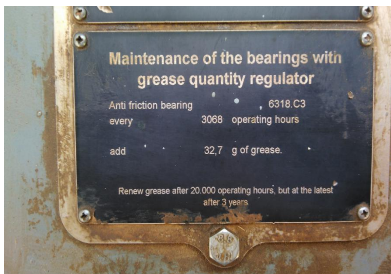
Figure 3 - This motor had a secondary plate reminding lube-techs which grease type to use.
