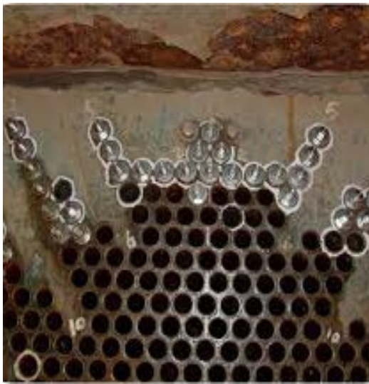
Figure 3 - Leaking tubes are identified and plugged
